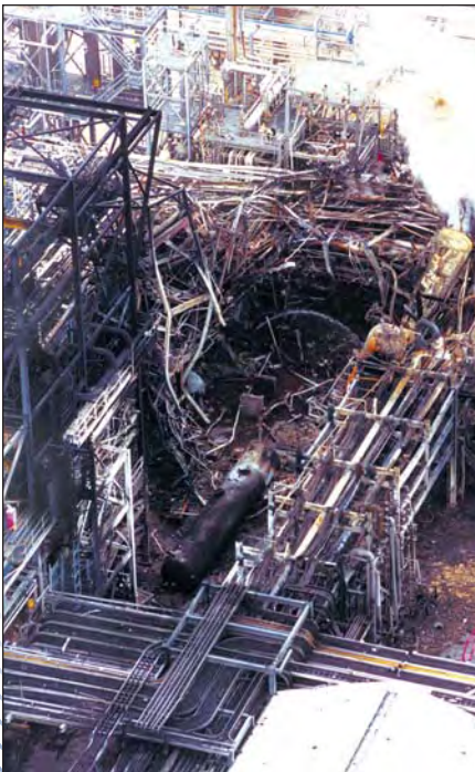
Petrochemical Plant Explosion
